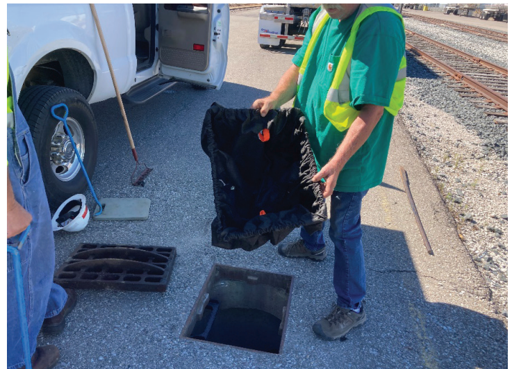
Picture of a typical filter bag being used in a storm sewer.
